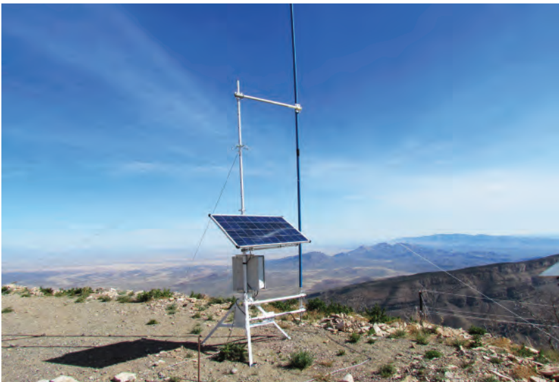
FIGURE 5 NGBPS C2 repeater station.
